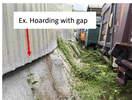
Photo 11 – Ex. Hoarding with gap along eastern boundary
