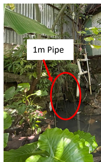
Photo 6 - Downstream Facility (Outlet 1m Pipe)
